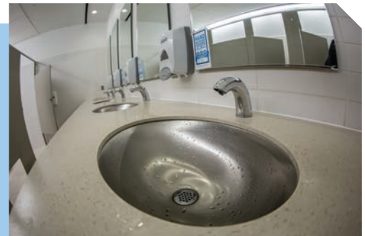
Low-flow water fixtures reduce GW's water consumption by nearly 30 percent.
