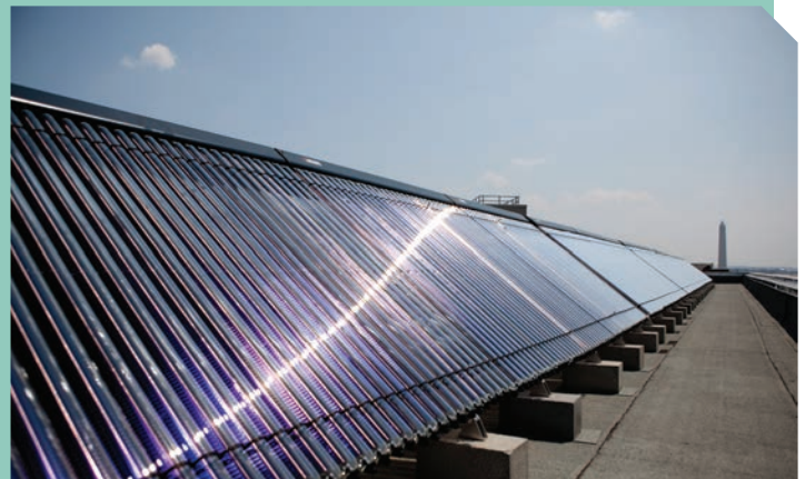
A rooftop solar thermal system in the heart of Washington, D.C.
