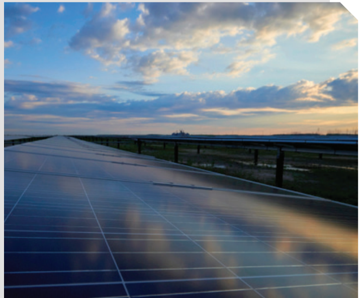
The Capital Partners Solar Project is a utility-scale solar farm in North Carolina.
